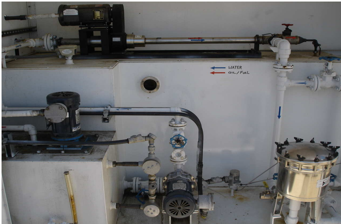
Figure 4 V-Inline 2000 Separator at Pt. Mugu
