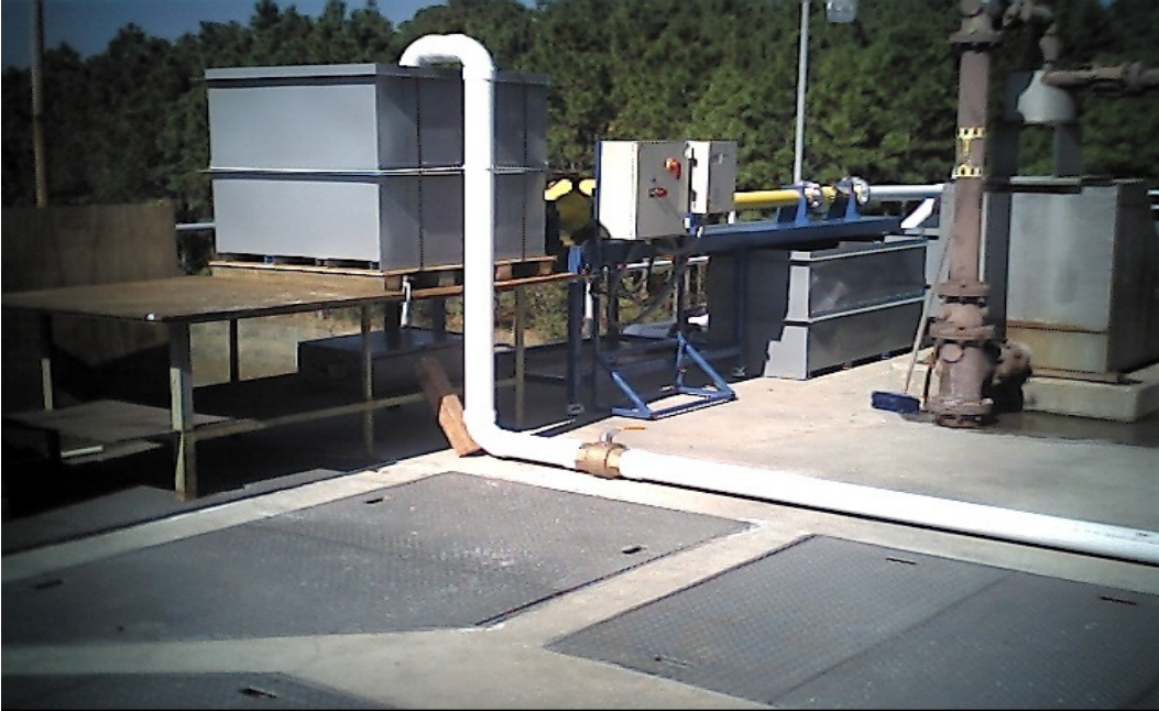
Figure 3 - View of Inlet Pipe and Equalization Tank Feed to Voraxial® Separator
